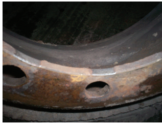
Worn wheel centre bore spigot
