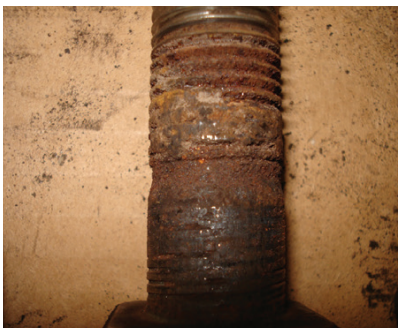
Corroded wheel stud
